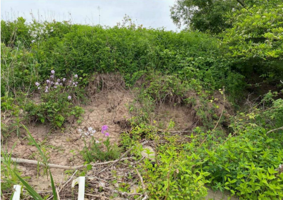
Figure 3. Photo of slope failure along the shoreline, Site 85/86
