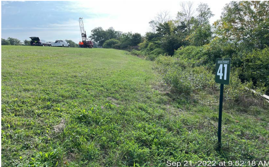
Photo 1 - Drill rig set up near crest of slope at Site No. 83. Photograph view toward south taken from NYSRHP dock site permit 41.
