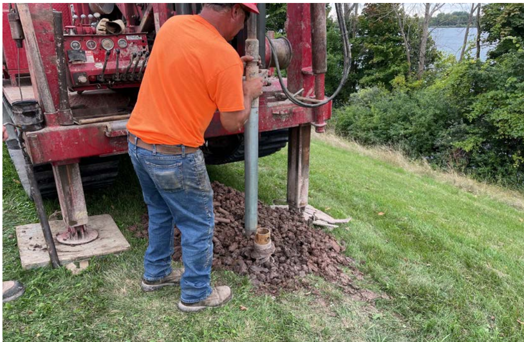
Photo 2 - Subcontracted drillers retrieving undisturbed (Shelby) tube sample from B-2 at Site No. 83.
