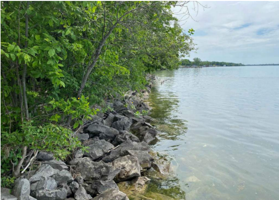
Figure 2. Photo of undersized rip rap, Site 83
