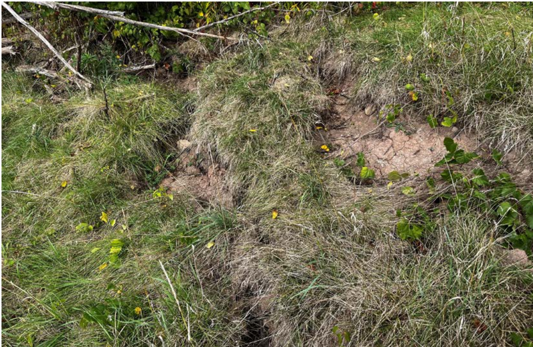
Photo 4 - Tension cracks observed in clay soil slope at Site No. 85+86.
